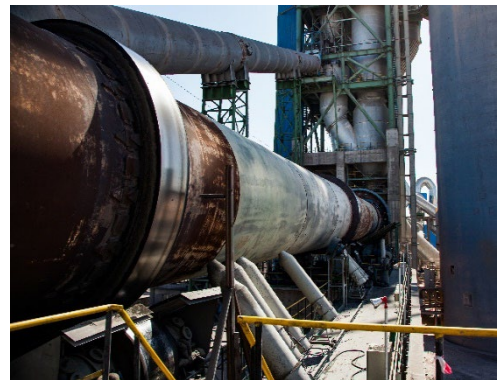
Cement plant gas furnace (rotary clinker kiln)
